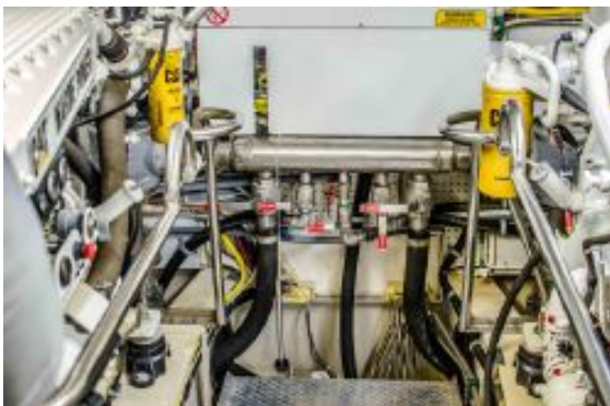
> SS water intake manifold steel lines fresh water engine flush system
