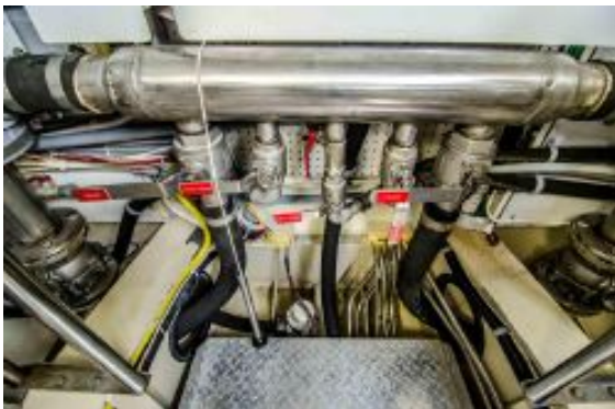
> Fresh/raw water engine flush
