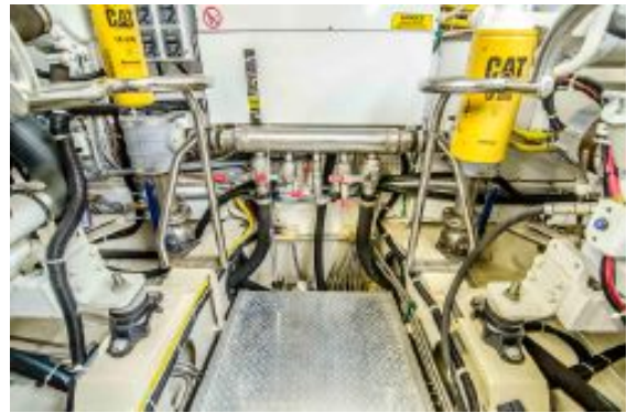
> Raw water manifold
