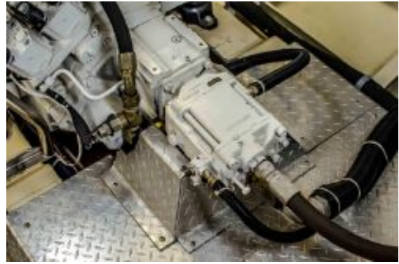
> Hydraulic pump off mains
