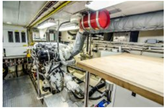
> Engine room work benches
