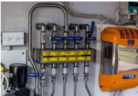
> Fuel polisher manifold SS lines
