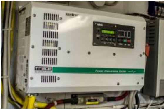
> Charles electrical system
