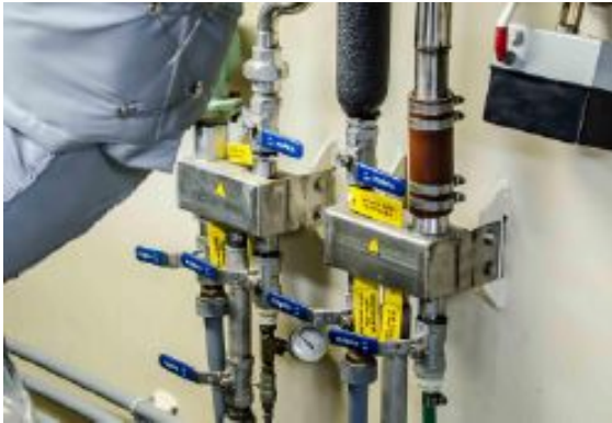
> Steel liquid lines
