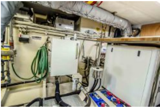
> Hydraulic fluid tank
